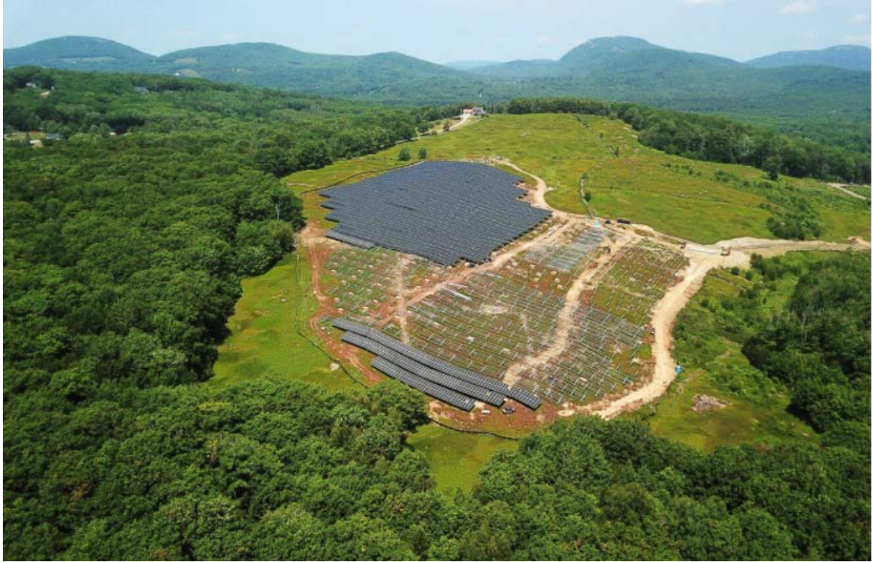
Figure 2. Aerial view of the solar array under installation. Photo credit: BlueWave Solar, CS Energy.
