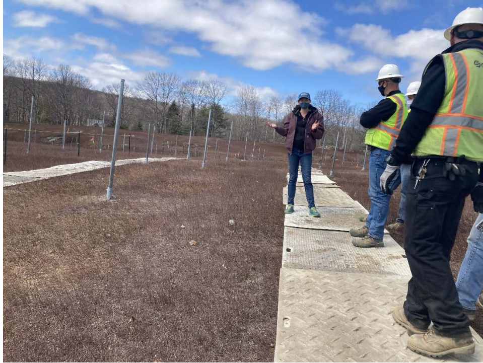
Figure 1 Dr. Lily Calderwood discusses impacts on blueberry plants with members of the construction and panel installation team. All are standing on the poly mats used to minimize disruption to existing blueberry plants in the Careful treatment. These mats were driven on by construction and installation equipment and served as pathways for workers. Photo credit: Brogan Tooley.
