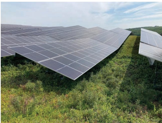
Research solar array installed above a wild blueberry field in Rockport, Maine.
